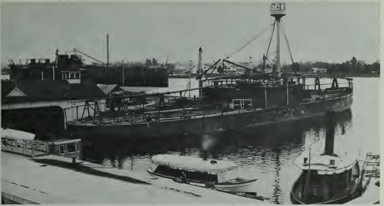
USS Amphitrite under construction at the Norfolk Navy Yard—The wood backing for the armor has been set in place but the belt is not yet installed. The tall military mast which was typical of the “New Navy” monitors has already been set in place.
